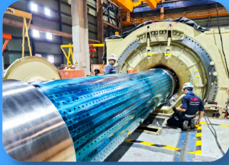
Maintenance Generator And Auxiliary " HITACHI " 330,000 kVA. 18,000 V. 2,860 A. 3,000 RPM.
