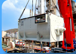
Disassemble, Overhaul, Rewinding, Assembly, Inspection, Dismantle, Installation Synchronous Generator 31,853 kVA. 11,000 V. 1,672 A. 1,500 RPM.
